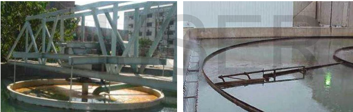
Figure 3: Effluent treatment plant
